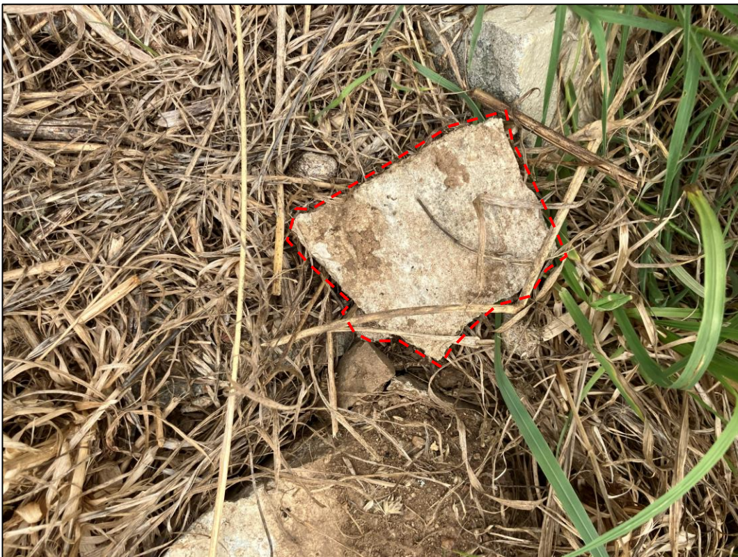
Site Photograph 13.3 Representative view of potential asbestos containing fibre cement fragment 'TP12-FC', as observed within on surficial soils south-east of the main residence, on 3 March 2026.
